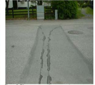
Figure 5: Fiber grooves on the pavement
